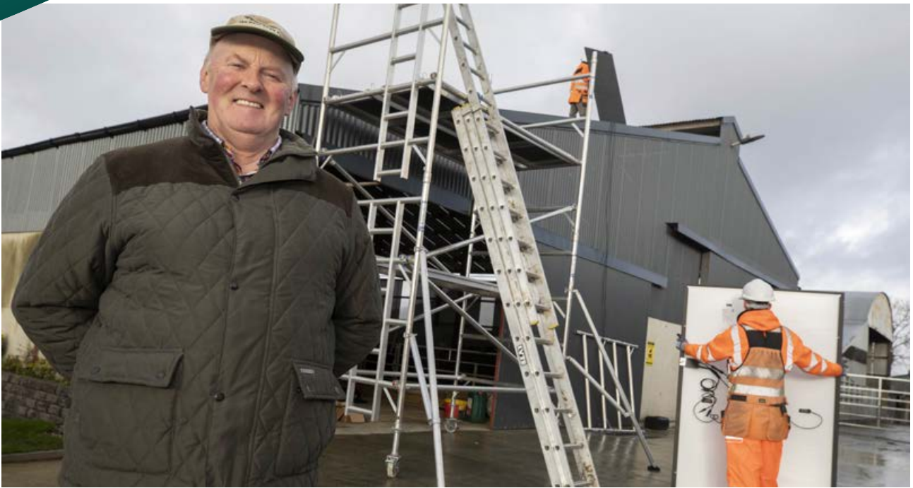
Poultry farmer Robert McBride at the installation of the solar panels on his farm in Corbeg, Co. Monaghan in December.
